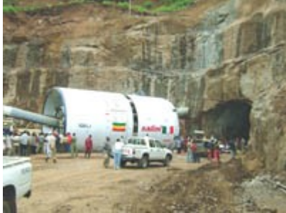
Gelgel Gibe II hydroelectric power plant
